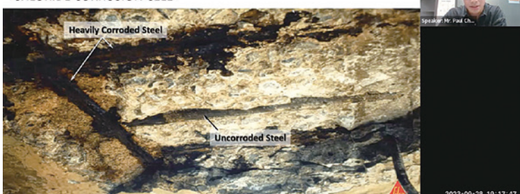
CHLORIDE CORROSION CELL
